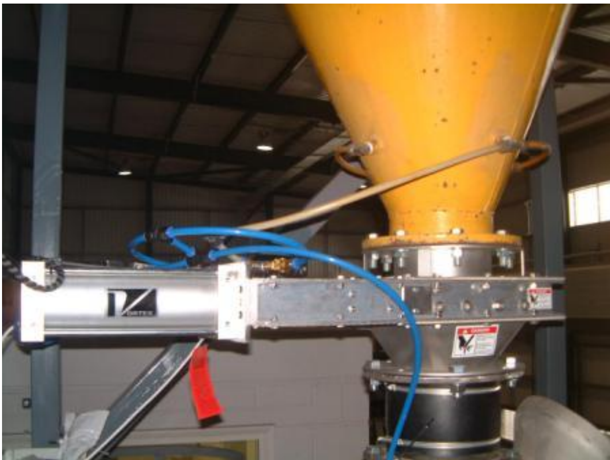
Vortex Roller Gate valve fitted to Wolfson’s pneumatic conveying test rig
