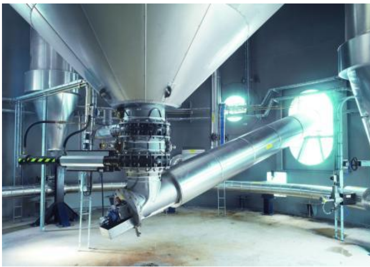
Van Beek screw conveyor beneath DRANCO hopper
