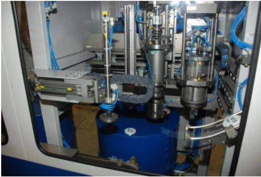
One of two fully automatic drum fillers at Suttons' St. Helens site
