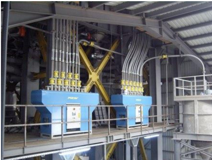
Twin batteries of 12-port multiport diverter valves from STAD
