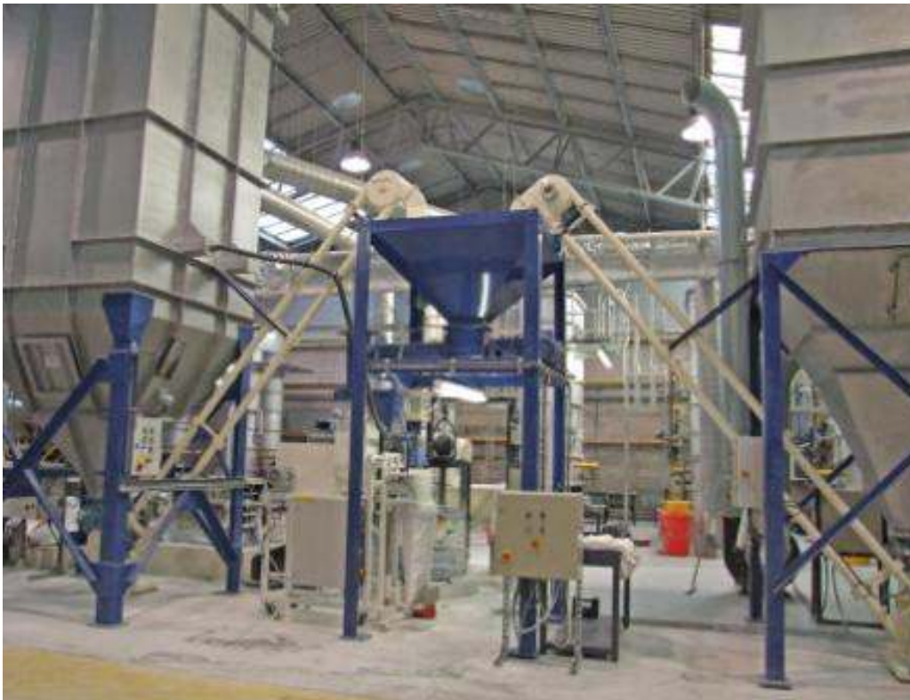
The latest two Spiroflow aero-mechanical conveyors at Keeling & Walker
