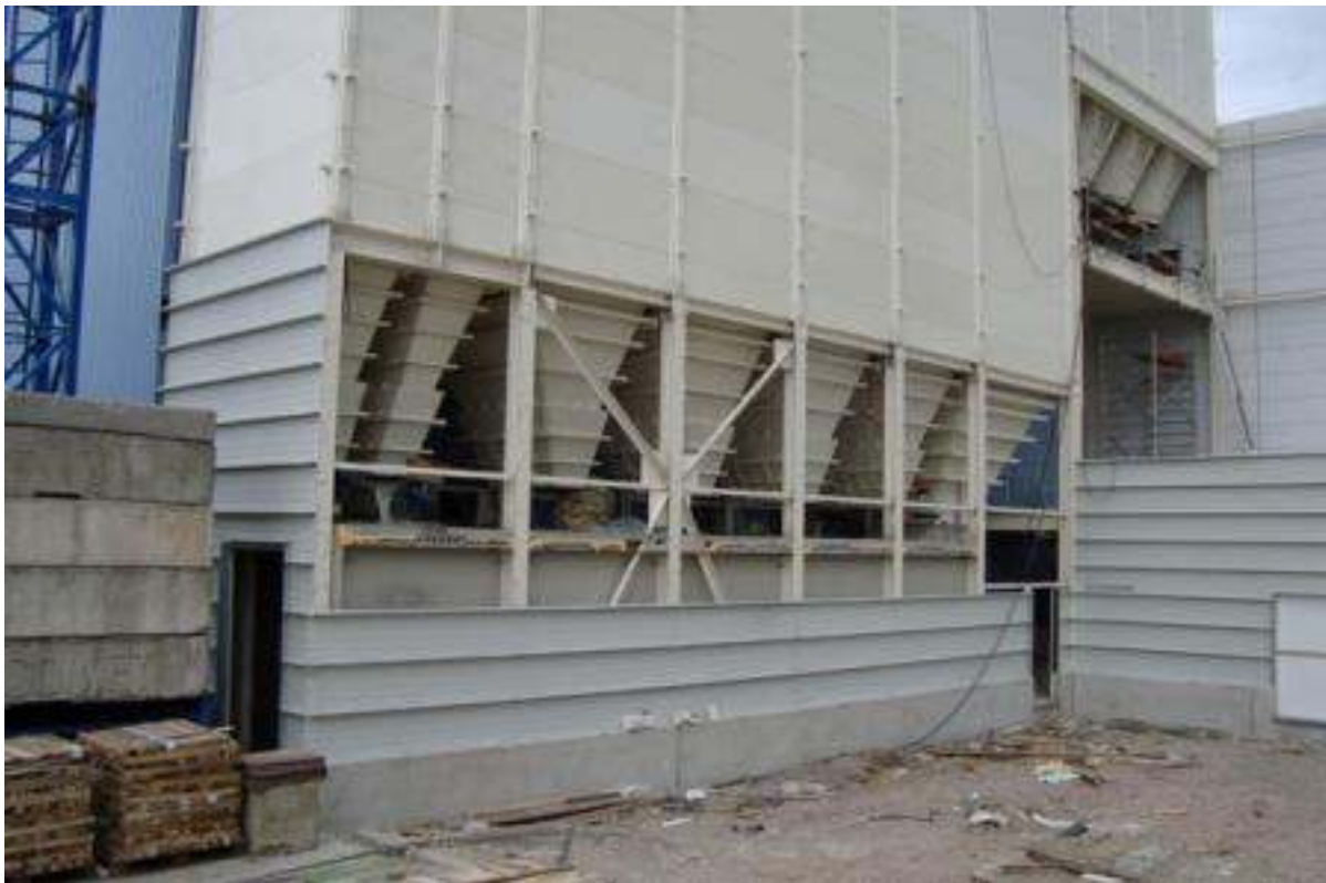
Extra SCE silo storage cells have been added to the Ostend production plant of Fides Petfood
