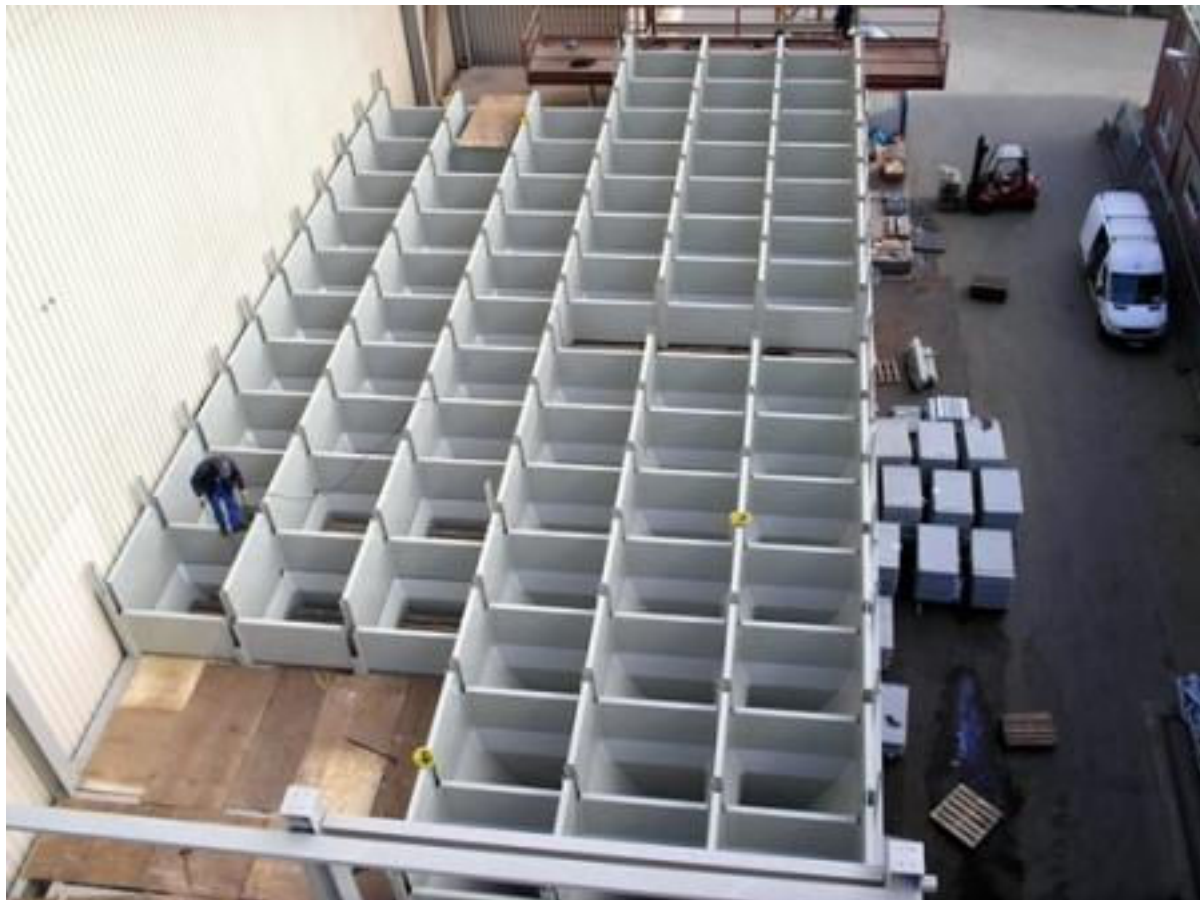
72 smooth-wall cells being installed by SCE Engineers at ATR's new bulk distribution station
