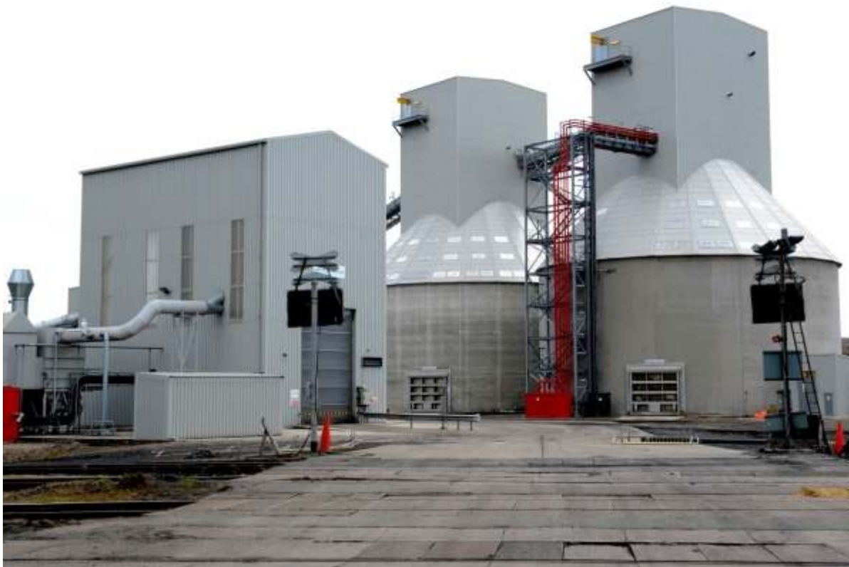
Typical biomass handling installation at a power plant where covered storage and enclosed conveyors pose a potential dust explosion hazard
