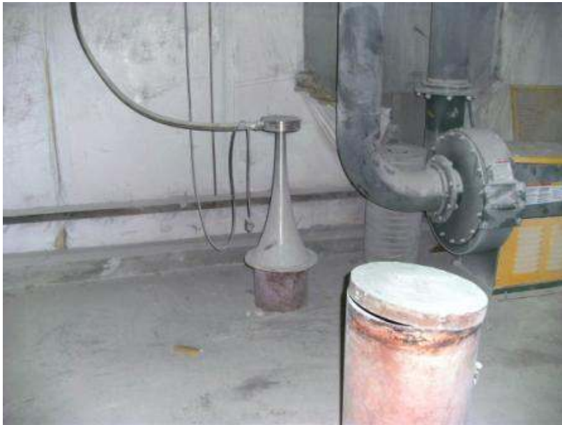
Primasonics acoustic cleaner at Ferro Corp
