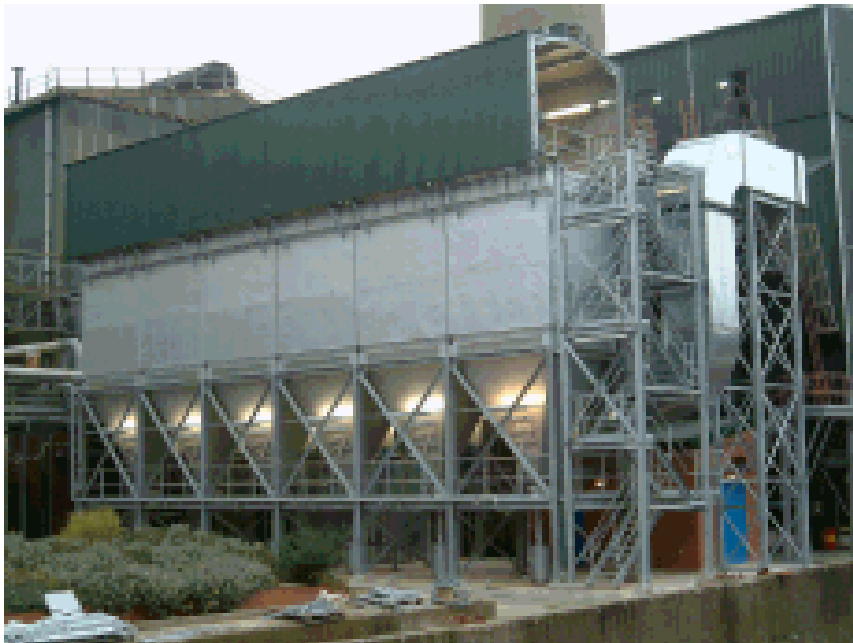
New baghouse installed by Pennaire Filtration
