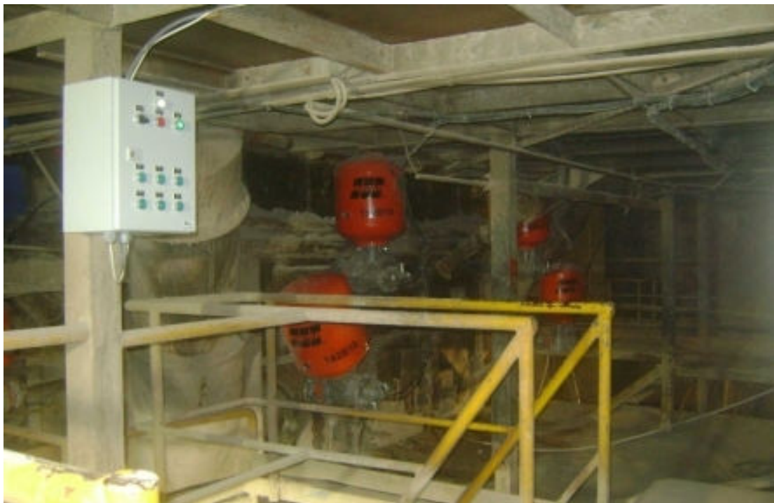
Martin Engineering air cannons at the Izmir Cimentas plant; the positive action of the Tornado valve amplifies output force by as much as 20% over standard air cannon designs
