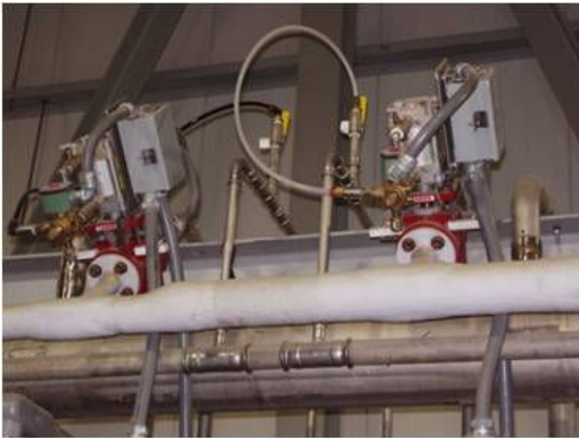
Larox Flowsys pinch valves fitted to a dry scrubber installation
