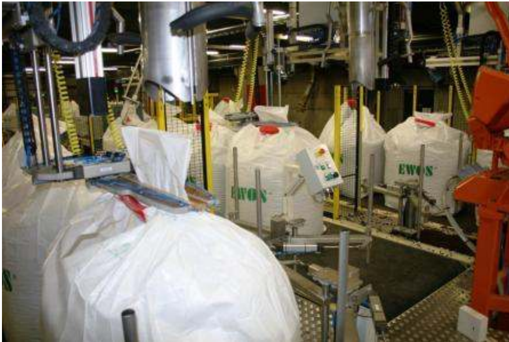
Three automatic PORTABULK bulk bag filling lines recently installed by Goodtech at the Floroe, Norway, plant of Ewos
