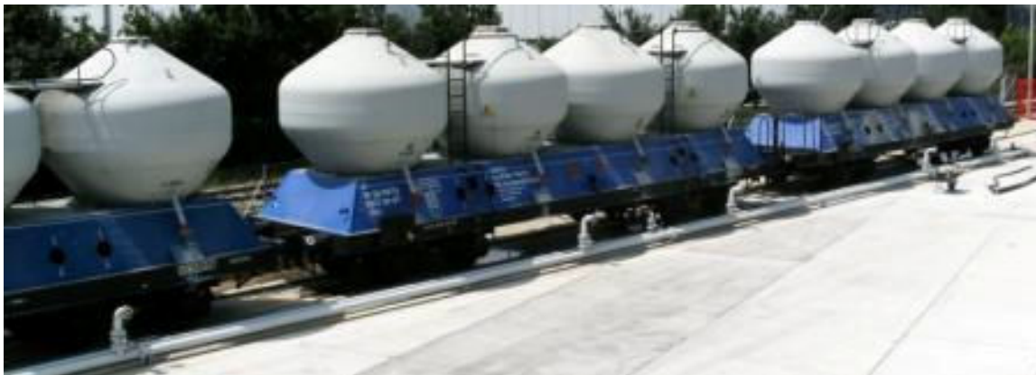
Pneumatic conveying installation at Transportbeton for unloading cement from rail tankcars
