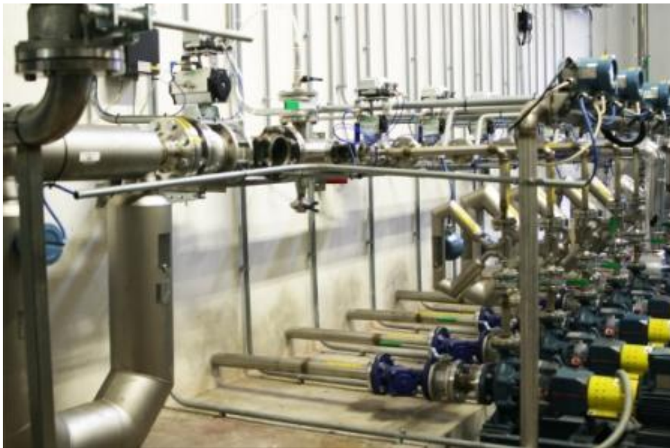
Emerson's Micro Motion Coriolis flow meters at the Faenza plant of Caviro
