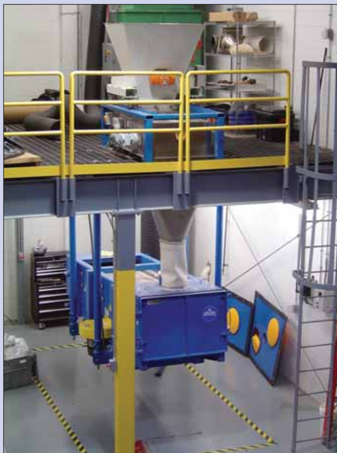
Sweco test plant showing GyraMax 300 gyratory sifter.
