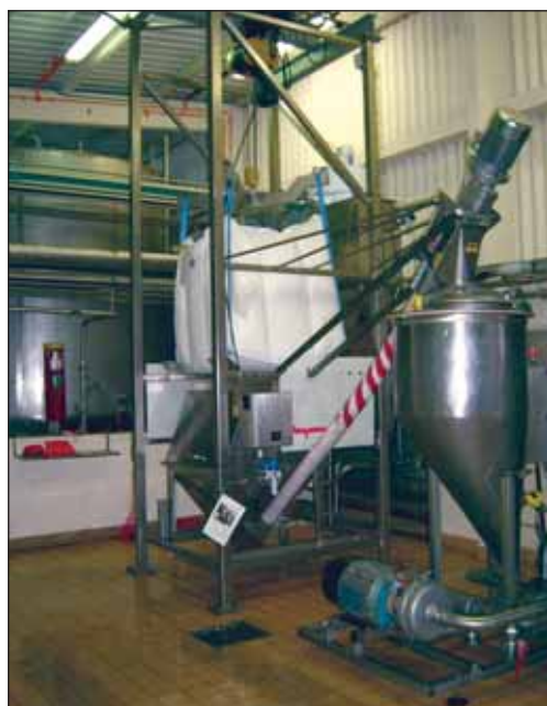
Flexicon food ingredient receival system at Danisco's Beaminster plant.
