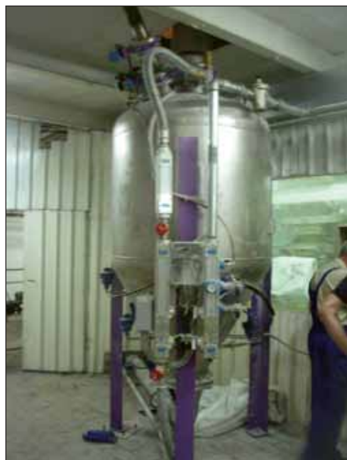
Pneumatic conveying specialist Air-Tec system of Italy recently installed an advanced positive-pressure pipeline system for handling sugar at the Lemarco refinery in Bucharest, Romania. This is described on p12 together with other similar installations, serving to illustrate the capabilities and advantages of positive-pressure conveying.
