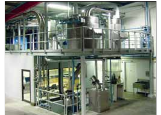
Dynamic Air's new test facility in Milton Keynes, UK.
