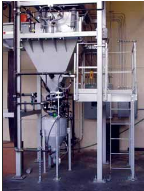
Dynamic Air HDP 4000 Full Line Concept dense phase system handles vermiculite for NOV ReedHycalog.
