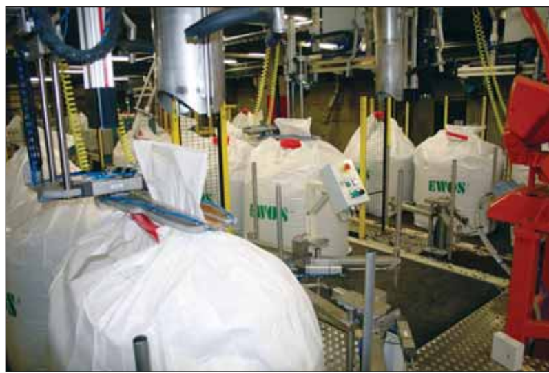
Three PORTABULK automatic FIBC filling lines installed by Goodtech at Ewos.
