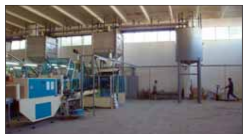
General view of Air-Tec system's sugar handling installation at Lemarco, Bucharest (see also front cover picture).
