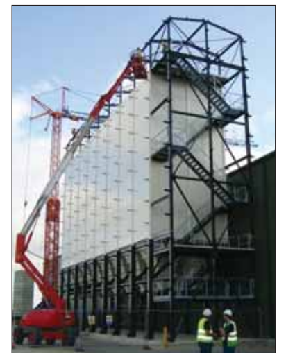
Working with GAME Engineering, SCE in 2009 installed this silo system for Wagg Foods in the UK.
