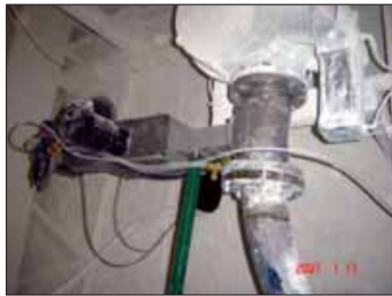
InterSystems sampler supplied by Wrights Dowson to ZChP monitors titanium dioxide at the upward bend of a pneumatic conveying line.
