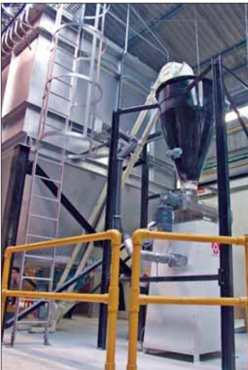
Spiroflow conveyor handling tin oxide.
