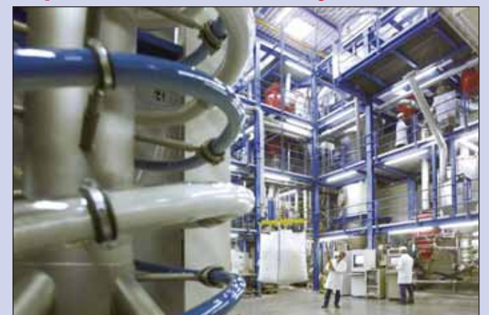
View inside Coperion's state-of-the-art Niederbiegen test plant where certain equipment combinations cannot be matched by any other test facility in the world.
