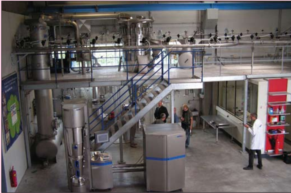
Ammag's test plant in Gunsirichen, Austria, offers advanced facilities for pneumatic conveying (dense and dilute phase), mixing and fluidised bed spray granulating trials.
