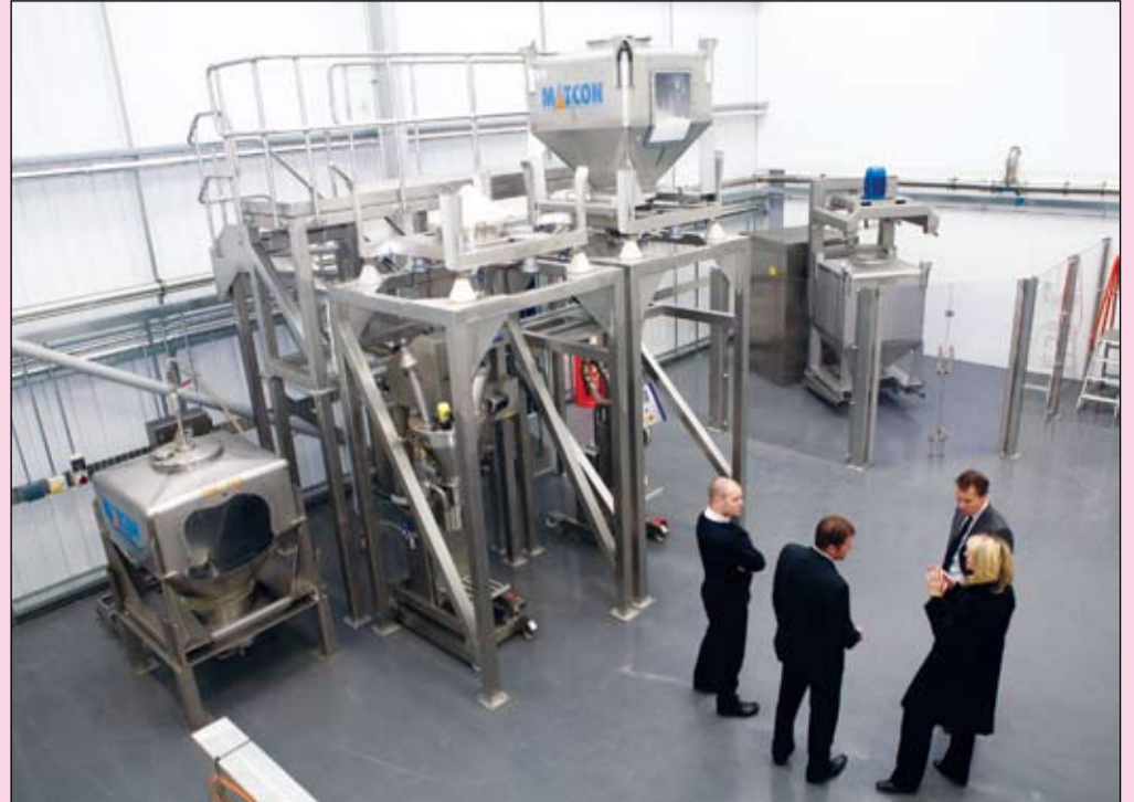
Matcon's UK test plant showing one of the company's IBC blenders and two of its different packing modules which are capable of catering for any pack weights and include sieving as well as metal detection capabilities.
