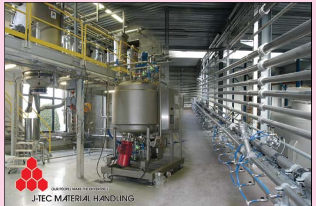
Part of J-Tec's Kapellen, Belgium, test facility where different gauges of pneumatic conveying pipework can be seen on the right.
